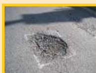
Potholes – this one in Myddleton Road is getting bigger and deeper by the week.
